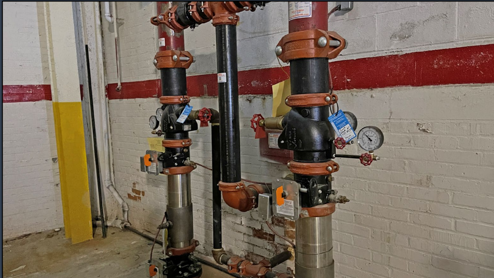
WET SPRINKLER SYSTEM
